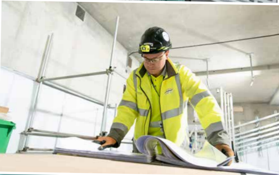
ELECTRIC PACE: Adam Hastilow surveys plans for the Electrical Building as supports, brackets and cable trays are installed (top).
