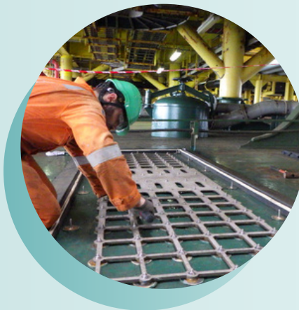
Transfer of stresses from the corroded structure to the new plate.
